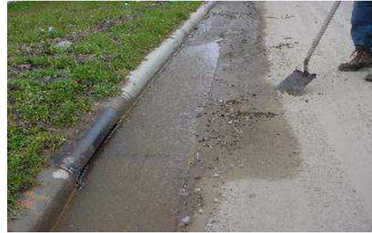
CAPTURED SEDIMENT IN GUTTER 12' FROM INLET
